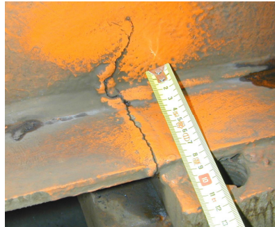
Figure 14 – Development of a weld crack
